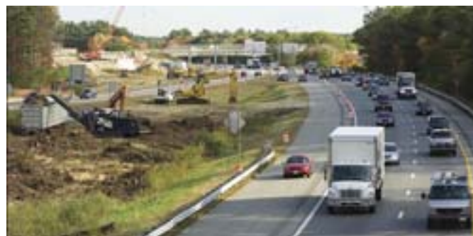
With University of New Hampshire Stormwater Center support, the New Hampshire Department of Transportation constructed two pilot gravel wetland treatments to help meet TMDL requirements for impaired waters as part of the Interstate 93 widening project.
